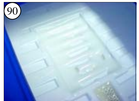
90 Put more of the filled epoxy into the motor base recess of the hull liner. Be generous.
