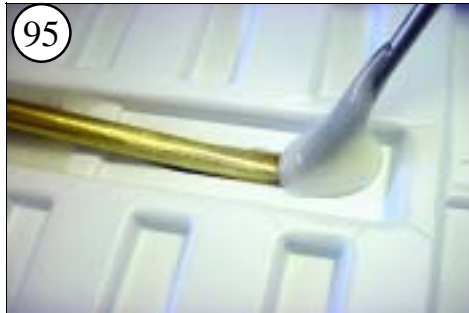
95 Add some of the filled epoxy to the recess around the stern tube.
