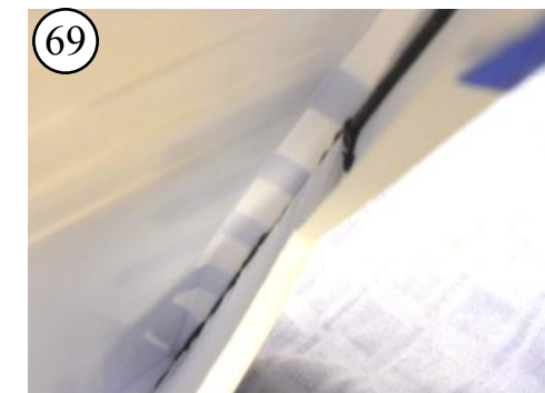
69 Where the groove stops, you can see the bead of sealant along the side.
