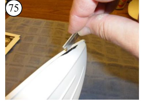
75 After the sealant has cured and the tape removed, any excess sealant can be removed by carefully cutting just the sealant with a hobby knife or razor.
